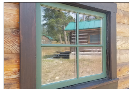
Fig. 7. Window at White Grass Ranch before the introduction of linseed-oil paint when waterborne latex paints were used, 2020. This window had early signs of paint failure, such as cracking and peeling, after two years. After 10 years, the paint had flaked off the bottom rail, portions of both stiles, and three muntins. This condition caused window glazing to fail in areas and required scraping and removal of loose paint, partial reglazing, and refinishing.
