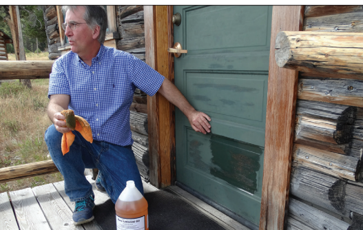
Fig. 6. A south-facing door at White Grass Ranch that was painted with linseed-oil paint has chalked after four years and is here being rubbed with purified linseed oil to refresh the paint film. Doors facing to the east, west, and north required re-oiling after eight years, 2016.
