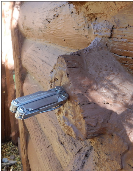
Fig. 3. Only a shell of waterborne paint is holding these decayed, hollowed-out log crowns together after decades of repainting with new waterborne latex and acrylic paint. Regular repainting without examining the condition of the underlying wood resulted in built-up paint layers that hid the wood decay, 2016.
