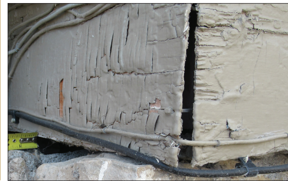
Fig. 5. Many painting campaigns have led to overpainting and a film thickness of around 1 millimeter in areas on this wood sill trim board, 2020.
