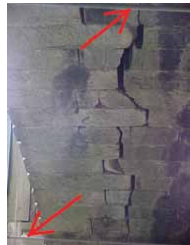
Fig. 5. Monocacy aqueduct, Montgomery County, Maryland, 1998. Arch barrel showing longitudinal cracks under the berm parapet prior to stabilization and restoration in 2010. Red arrows indicate two of the temporary tie rods, which were installed under the arches to arrest the transverse movement of the spandrel walls and barrel arches; note also that the cracks are wider at the apex. Photograph by Denis McMullan.
