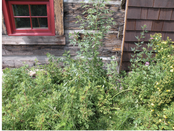
Fig. 4, bottom left. Deterioration of exterior millwork caused by trapped moisture. Photograph by Ronald W. Anthony.
