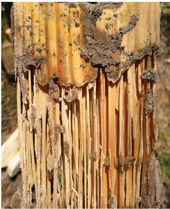
Fig. 2. Damage to untreated wood caused by termites after only six months of soil contact in Louisiana. Courtesy of Stan T. Lebow and the U.S. Forest Products Laboratory.
