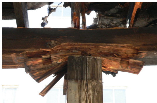
Fig. 1. Advanced decay of a timber girder and bearing plate. The deterioration was caused by years of exposure to roof leaks and resulted in the bearing plate being crushed. Photograph by Ronald W. Anthony.
