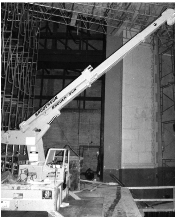
Fig. 7 Planning for some historic-preservation projects must include scheduling multiple trades. In this theater project, the schedule required plaster and paint work to occur at night while a new orchestra pit was constructed below during the day. Dust control, equipment emissions, scaffolding design, and worker schedules were all part of the plan developed by the project team. Photograph by the Christman Company.
