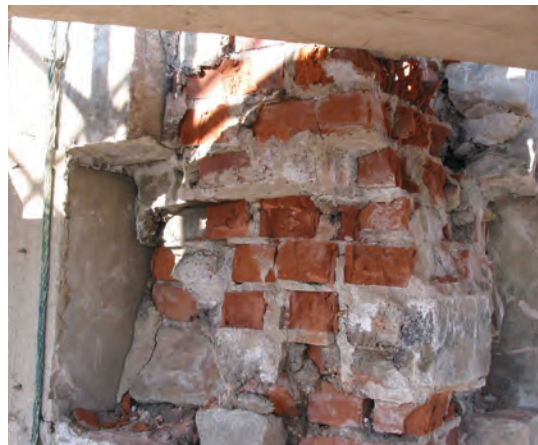
Fig. 2. Brick failure at Saint Paul's Church, Cranston, Rhode Island, 2002. This mass brick masonry was set with a portland-cement mortar that has failed due to decades of water infiltration and freezing and thawing. It is an example of the type of non-sacrificial global assembly failure that occurs with more modern, higher-strength mortar binder materials.
