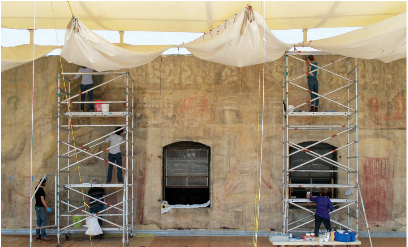
Fig. 3. The GCI conservation team performing cleaning during the 2012 treatment, which also included fills of cracks and losses, removal of tar staining, and limited aesthetic reintegration. Tar stains can be seen along the lower edge of the mural as intermittent dark spots. Photograph © J. Paul Getty Trust.
